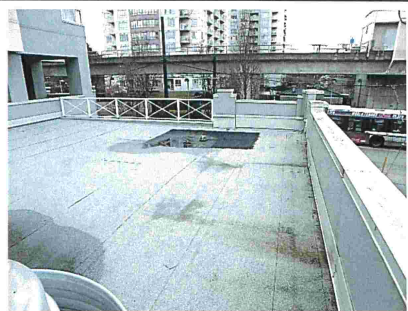
Photograph 16: Tower View of the lower flat roof on floor level 2 (Looking North).
