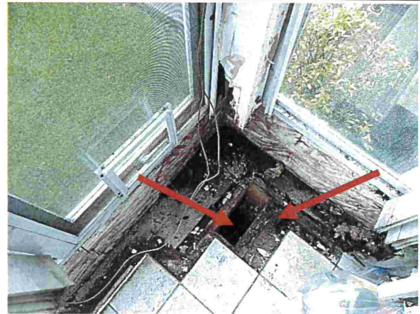
Photograph 27: Town Homes (#3362) The left arrow points to a hole after removal of some of the decayed plywood floor board. The right arrow points to a decayed floor joist.
