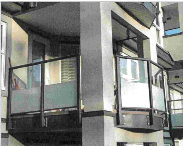
Figure 3.11 Aluminum-framed guardrail with clear and opaque glass panels.
