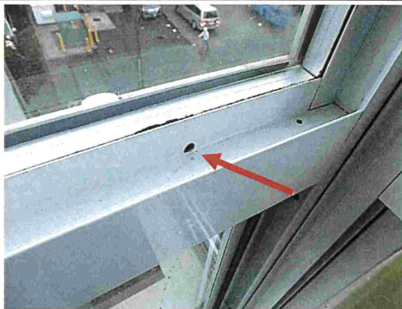
Photograph 32: Tower (#303) The arrow points to an example of a weep-hole drilled (by other parties) into the window frame to drain water that accumulates in the upper horizontal trough of the frame. Similar weep-holes were added to other window at other units in the tower.
