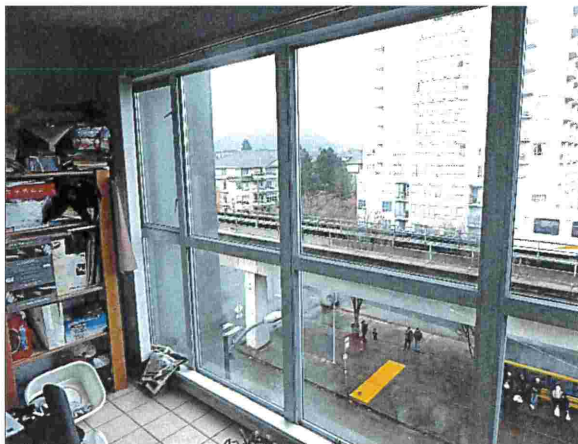
Photograph 9: Tower View of a typical "window wall" at an enclosed balcony (North elevation).
