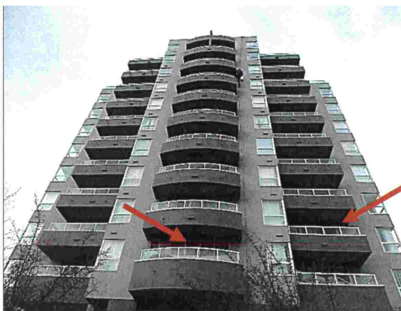
Photograph 11 Tower The arrows point to the typical outdoor balconies exposed to the air (South elevation). See Photograph 12 .
