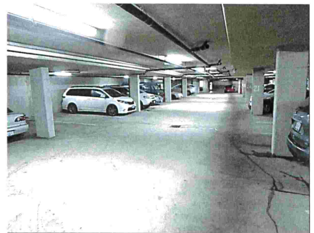
Photograph 24: Parkade View of the residential Strata Owners' parking area in the below-grade parkade.
