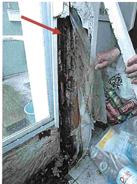
Photograph 28: Town Homes (#3362) The arrow points to a decayed column. The extent of decay continues higher than the arrow.
