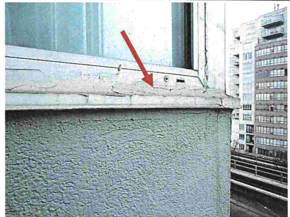
Photograph 43: Tower .The arrow points to caulking at exterior joints of a typical window. The caulking appears weathered.
