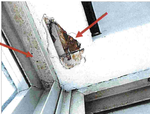
Photograph 40: Tower (#1006) View at the ceiling above the windows in the enclosed balcony. The left arrow points to water stains from previous condensation along the head of the window frame. The right arrow points to corrosion on the metal components behind the interior drywall assembly.
