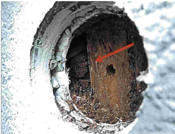
Photograph 50: Town Homes (#3362) EO made at the North elevation, on a narrow East facing wall at floor level 2, below a horizontal joint. The arrow points to decayed plywood sheathing board.
