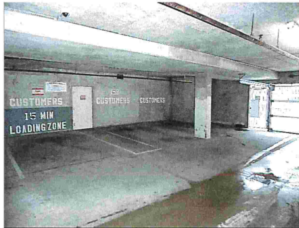
Photograph 23: Parkade View of the Retail / Commercial parking area in the below-grade parkade.
