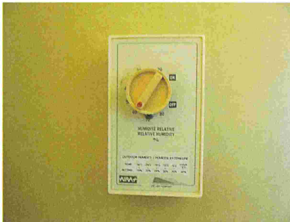
Photograph 38: Tower (#901) View of the wall mounted humidistat control typically located in the living room.
