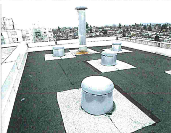
Photograph 15: Tower View of the flat roof on the Mechanical Penthouse. See Photographs 14 & 16 .
