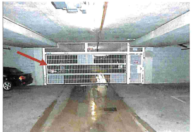
Photograph 22: Parkade The arrow points to the interior lift gate which provides access to the residential Strata Owners' parking area in the below-grade parkade.
