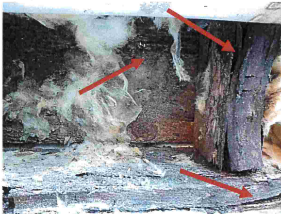
Photograph 30: Town Homes (#3376) The top arrow points to the decayed wall stud. The middle arrow points to decayed plywood sheathing. The bottom arrow points to a decayed wall plate. See Photograph 29 .
