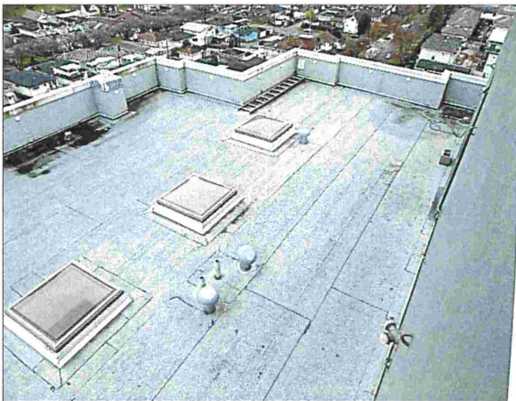
Photograph 13: Tower View of the upper flat roof at the top of tower. (South side of Mechanical Penthouse looking West)
