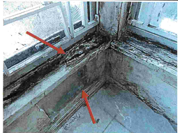
Photograph 29: Town Homes (#3376) The left arrow points to fungal growth and severe decay of the wood stool plate. The right arrow points to the location of the EO in the interior drywall. See Photograph 30 .
